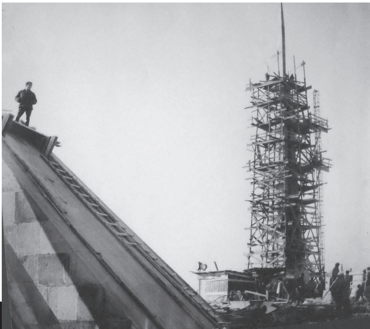
Construction of the memorial for the victims of the Genocide of Armenians in 1915 in the Ottoman Empire (1965-1967)
